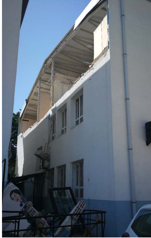
Fig. 3 Raised floor constructed with structural steel and truss-beam roof cover, insufficiently connected to the masonry wall parapets.
