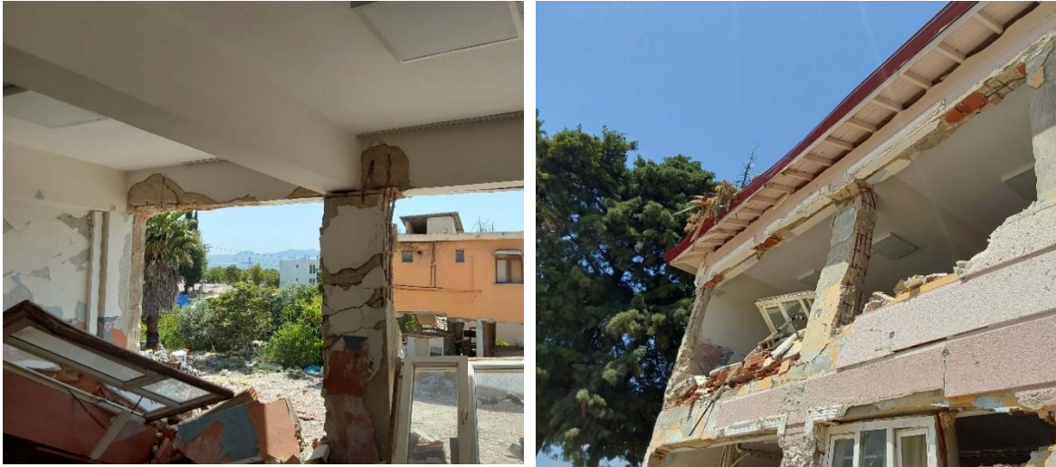
Fig. 6. Column top sheared-off at the construction joint, due to pounding from a (collapsed) adjacent structure: internal and external view (from left to right).
