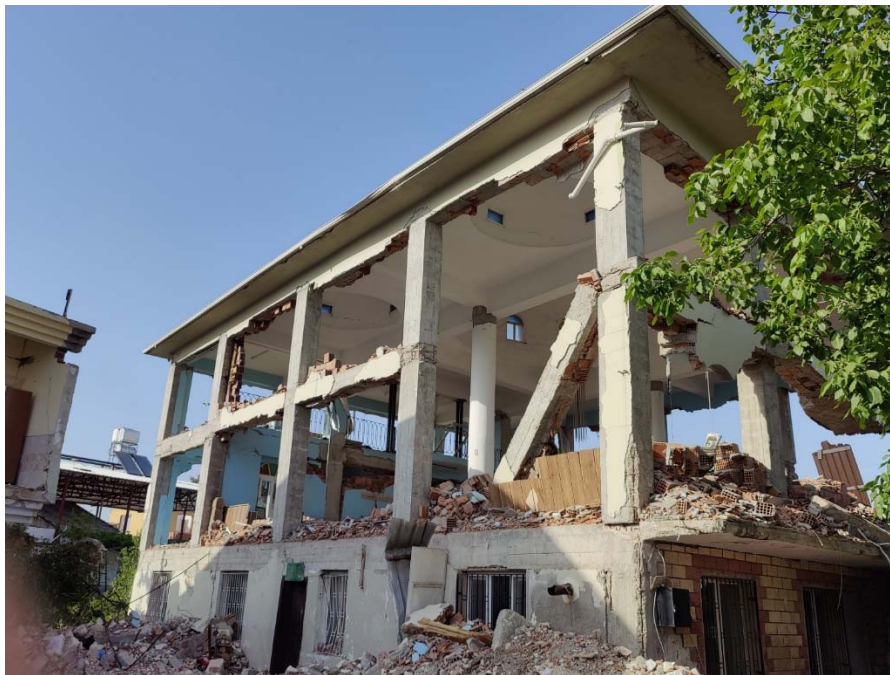
Fig. 8 Partial collapse of RC beam and floor slab.
