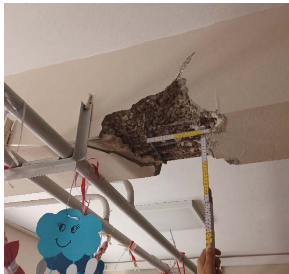
Fig. 3. Local damage in a ground floor beam, at about one-third span's length away from the nearest supporting column, at a point where heating pipes are suspended from the beam's web. Damage most probably attributed to bad quality concrete (presence of large voids and lack of hardened cement paste) and (likely) interaction with the pipe.
