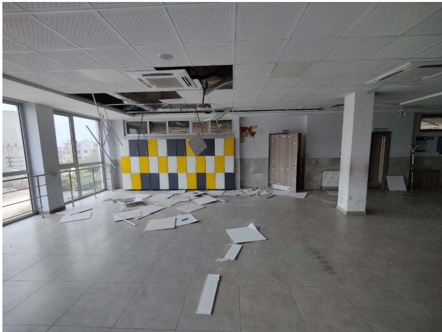
Fig. 7 – Front view of the building and fallen suspended roof panels.
