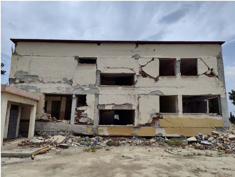
Fig. 4 – Prospect view of the building exhibiting widespread damage (no documented pre-earthquake retrofit).
