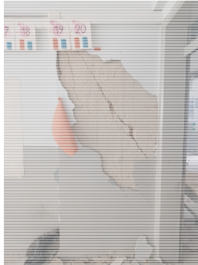
Fig. 2. Shear failure of an RC wall at the ground floor.
