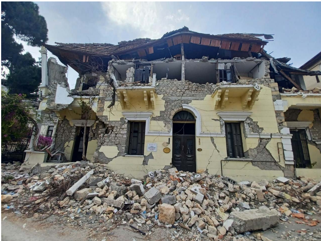
Fig. 9 - Damage state of a stone masonry building in the historic city-center of Antioch: collapse of the roof, in-plane and out-of-plane failure mechanisms of the masonry walls. The cantilevers of the balconies overlooking the main entrance have survived, oddly enough.
