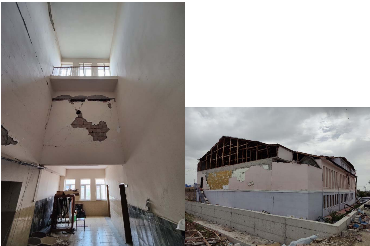
Fig. 6 – Front view of the building, flexural cracking of a beam, damage of the masonry infills and damage to the roof cover.
