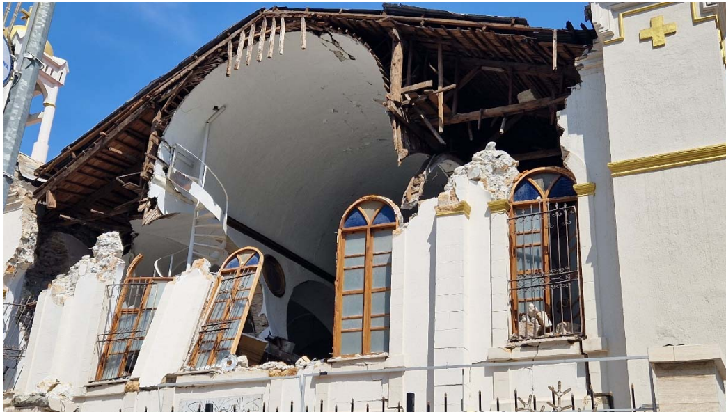
Fig. 11 – Collapse of the frontal wall of a masonry church with a wooden roof.
