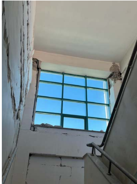
Fig. 14 – Damage encountered in the existing structure.
