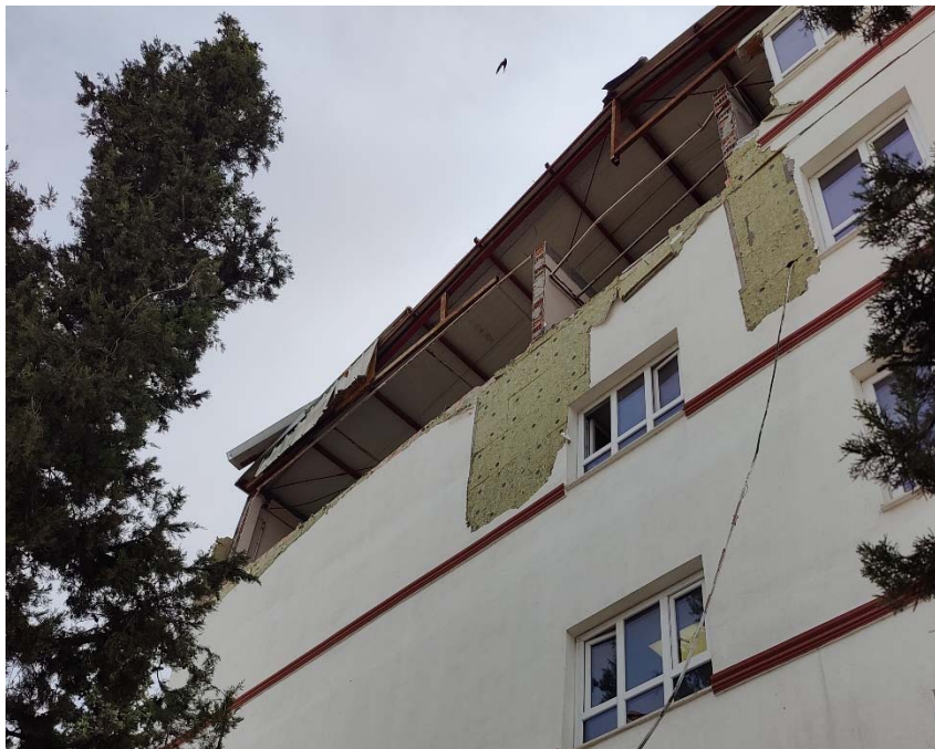
Fig. 5 – Front view of the building; out-of-plane collapse of the top floor’s masonry infills (building retrofitted via addition of shear walls prior to the seismic sequence).
