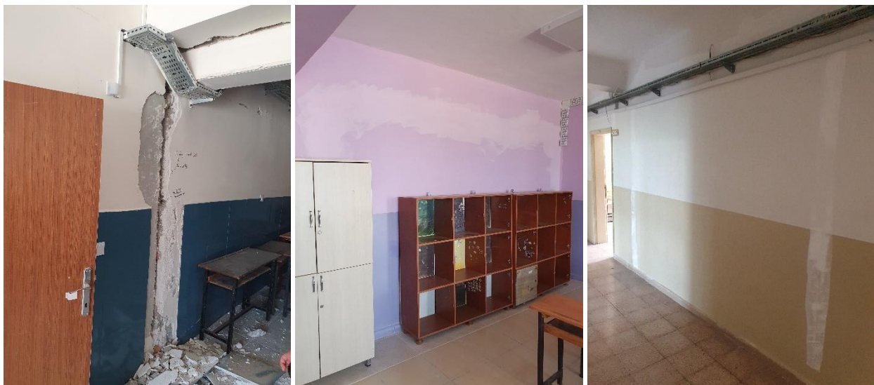
Fig. 8 – Visible damage due to pounding between the different structural units across the expansion joint (a), and cracks along the interface between original RC frame and additional shear wall adopted as retrofit measure (b, c).
